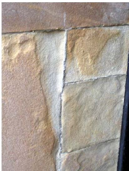
Accelerated decay to the sandstone at the front entrance porch from waterborne chemicals passing through the core of the wall at the west elevation – compare with the photograph taken in 1973 (page 70) (Photo: author)
