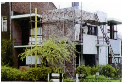
Below: the Schröder House under repair, showing the original brick core to the walls (from the Brick Bulletin )
