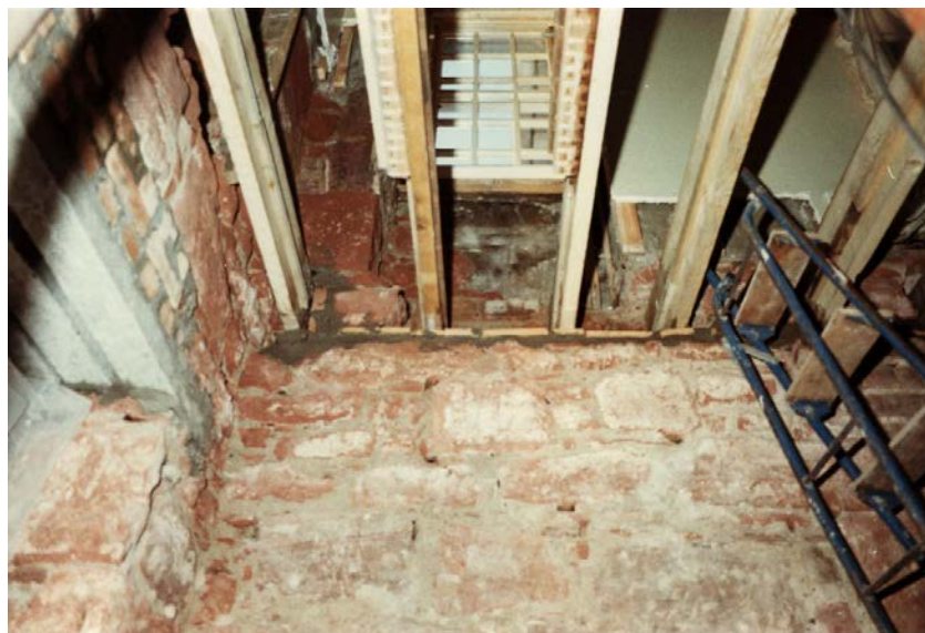
Consequences of a dry rot outbreak in the southwest corner of the Dining Room showing affected joist ends cut back and timber safe lintols replaced in precast concrete © NTS
