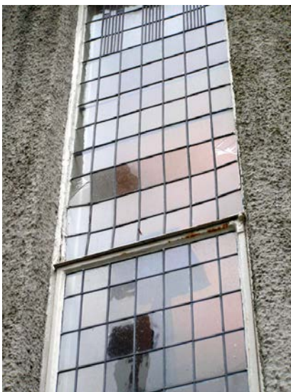
Above: windows at The Hill House of varying patterns and materials, of timber, steel, lead and glass – although they may be unconventional in design, they are capable of being repaired by orthodox conservation techniques without causing major intervention or the replacement of original material (Photos: author)
