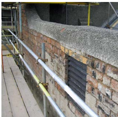
The parapet to the south elevation of the School of Art, in the course of being repaired in November 2011
