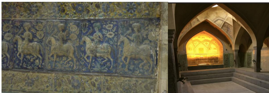
Tiles installed in the Hammam-I’ ali Quli Aga , Isfahan, c. 1850-70 (Picture credit: Moya Carey)
